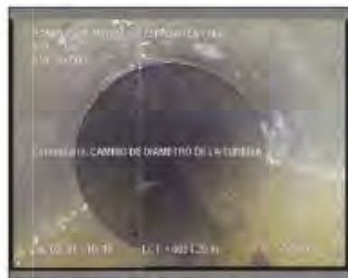
Foto: 11_1_5_28022021_101304_A.JPG 24,7m, Comentario
